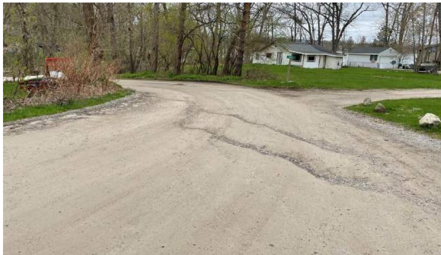
Figure 4 – Rilling of Existing Gravel Roadway
